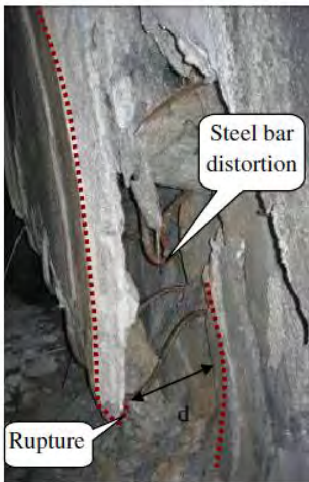
a) Lining rupture
