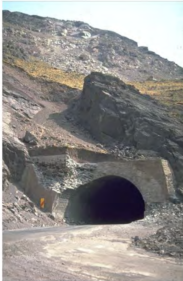
Figure 4: Tunnel portal damaged by rockfall during the 1990 Manjil earthquake
